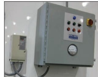
CONTROL PANEL WITH VFD
